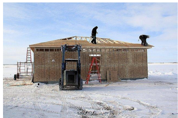
Before the year ended, basic framing for the Cottage Washroom and Maintenance Building was completed
